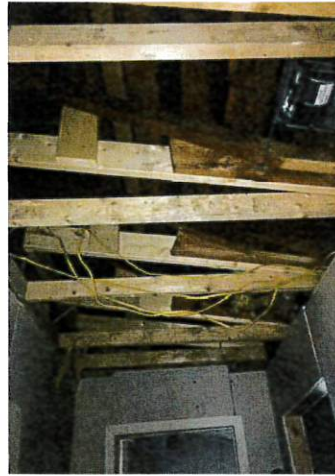
Exposed ceiling / no lighting
