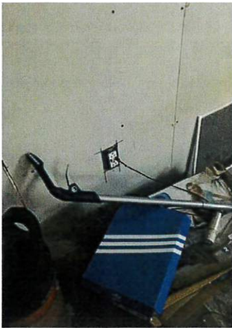
new unpermitted electric work
