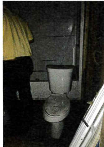
toilet not hooked up - only bathroom
