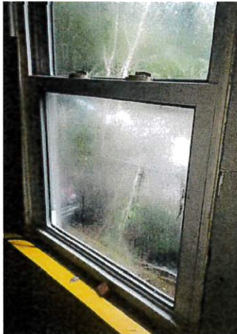
cloudy windows - not sealed.
