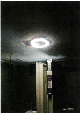
improper light, storage of new building materials
