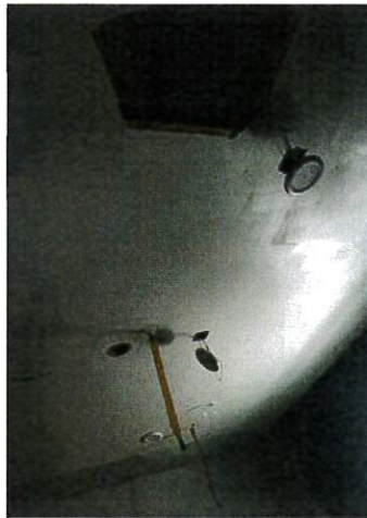
dangling light fixtures
