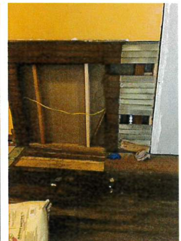
Open wall from former chimney?
