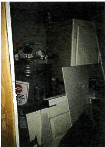
blockers & imperable water heater
