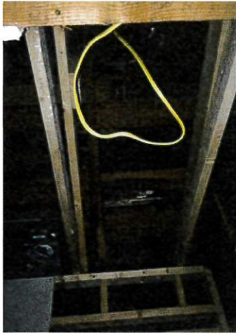
Exposed studs / wiring
