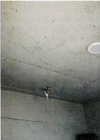
moisture spots on unpainted drywall
