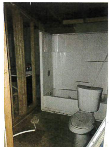
no bath fixtures connected
